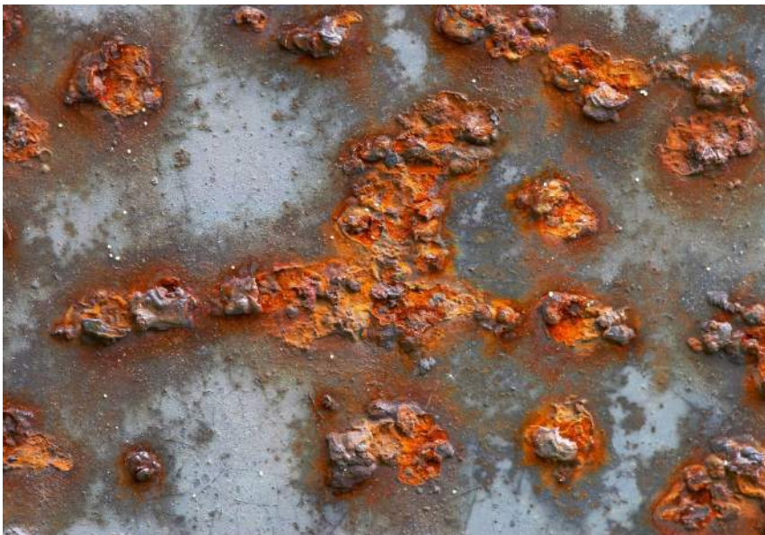
Example of detrimental effect of soluble salts (surface corrosion)
